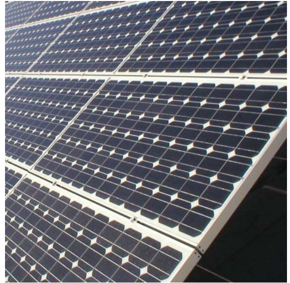
Photovoltaic Solar Electric System
